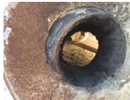
After 2 months in service, a competitor's valve showed signs of upstream severe media buildup — causing frequent leaks and lockups.
