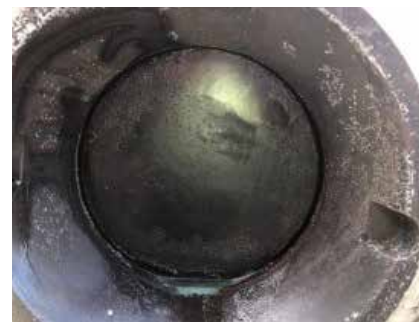
After 18 months in service with no issues, the valve showed no signs of wear or upstream media buildup.
